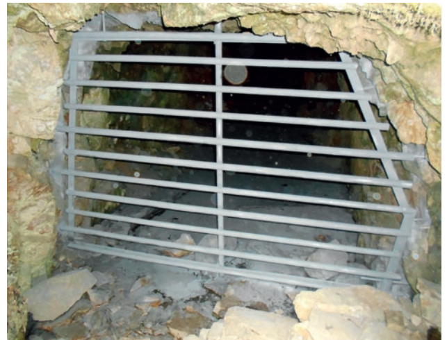
The grille is used to secure the entrance to a former mining gallery, sized to allow the bats to pass through
